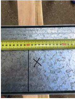
Set-out "E" for joist brackets @ 450 c/c. Place a cross "X" on the side the joist will go.
