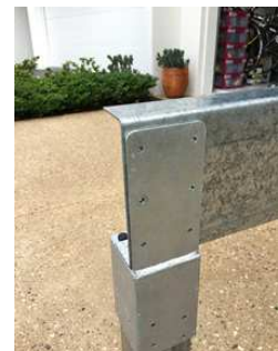
"D" bearer section ready to be fixed to "C" with "J" Tek's.
